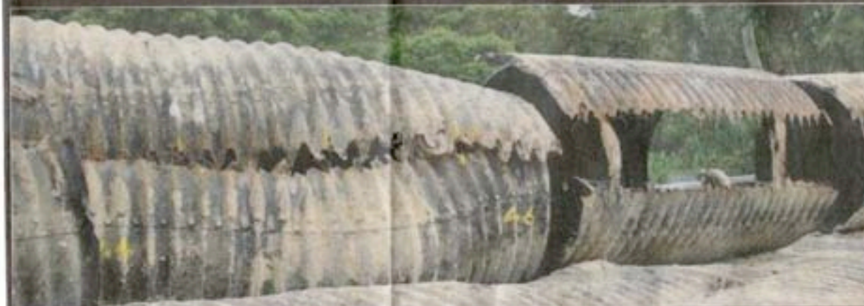
Maintenance concerns ... rusted-through corrugated steel pipes that supported the Pacific Highway at Piles Creek.
